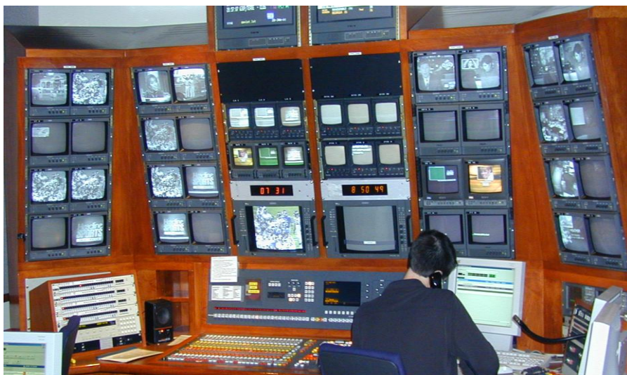
Master Control room at CNN
